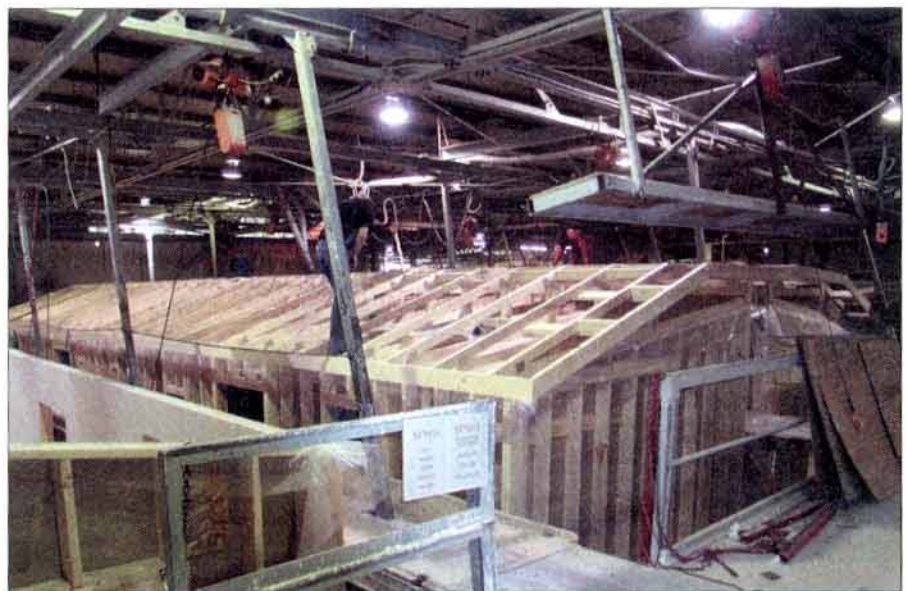
After assembling the roof on a side table it is hoisted and set onto the home using overhead cranes. Trusses are engineered and built to rigid government snowload specifications.
